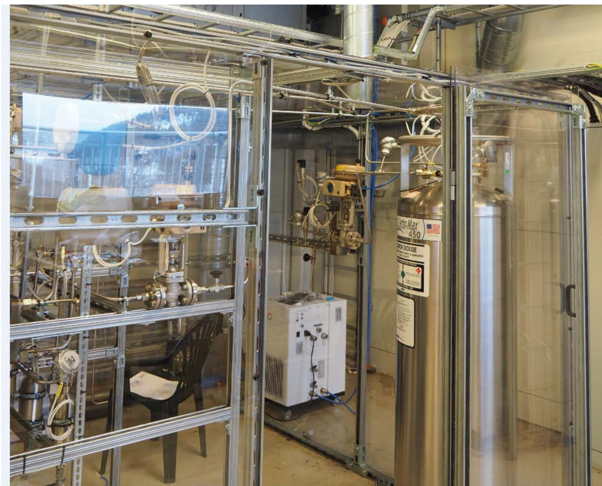
Figure 2-5 Cabinet housing the CCLU. The Lauda cooler is the white unit in the middle, and the Carbo-Max storage tank to the right.
