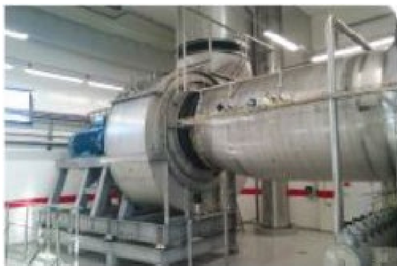
Figure 3.2.1. Flue gas centrifugal fan
